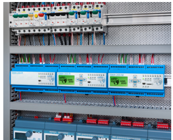
GMA200-MT with two relay modules GMA200-RT and GMA200-RTD mounted in a control cabinet.
